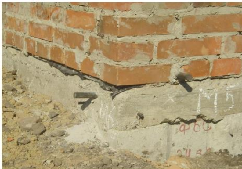
Fig. 2. Surface wall marks on the basement of the bearing walls of the object of geomonitoring for fixing sediment
