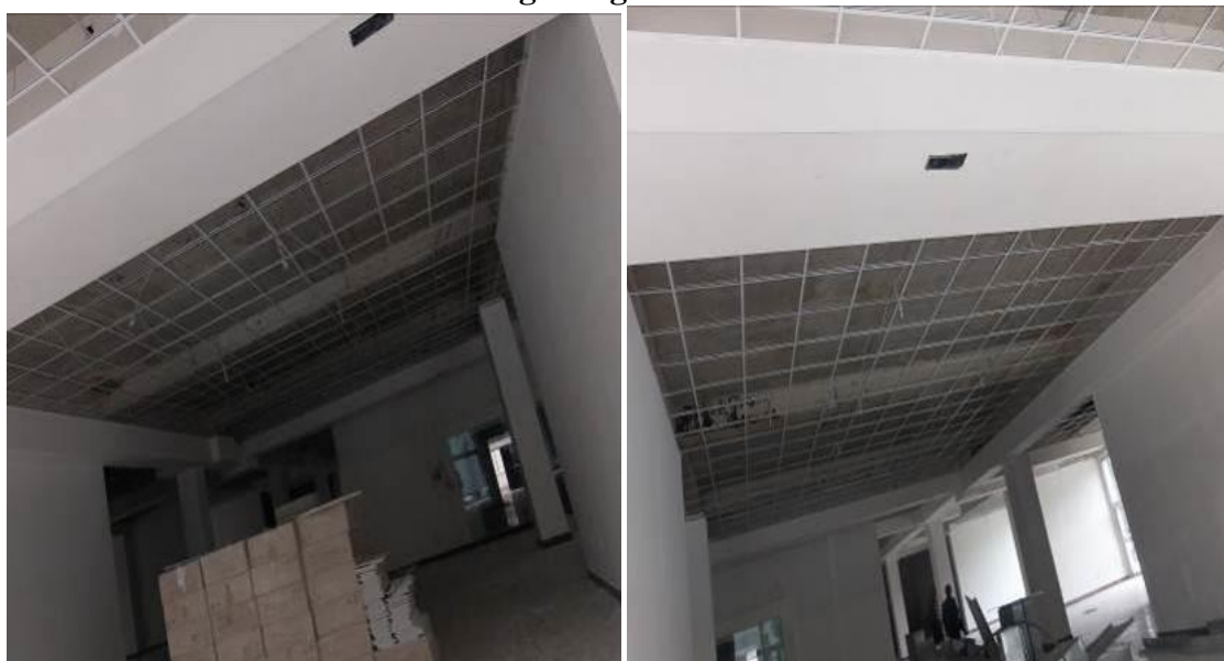
Fig. 6. The nature of the propagation of cracks in the crossbars of the first floor of the building along the V-D axes
