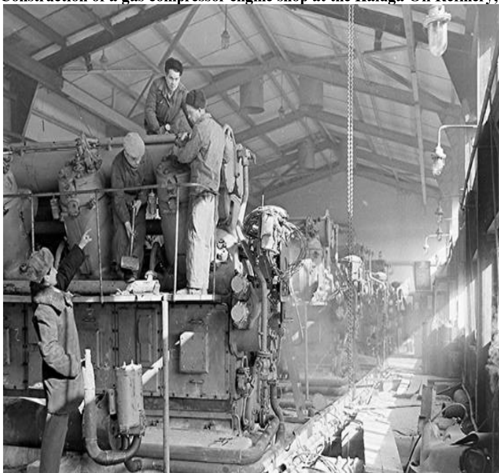
Figure 2. Construction of a gas compressor engine shop at the Kaluga Oil Refinery, 1957
